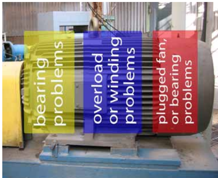
Figure 1. AC motor heat diagnostic pattern.
